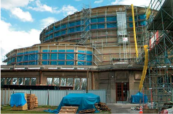
Ryc. 3. Widok Hali Stulecia w trakcie remontu w 2009 roku Fig. 3. View of the Centennial Hall during renovation in 2009
