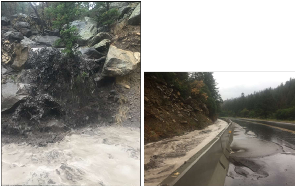
Figures 3.5. Left: view looking upstream at a gully on the east side of U.S. Highway 64. The gully originates at the high burn severity area in Midnight Mesa. Right: view looking downstream of the gully at the flow being routed by concrete wall barriers to a road culvert.
