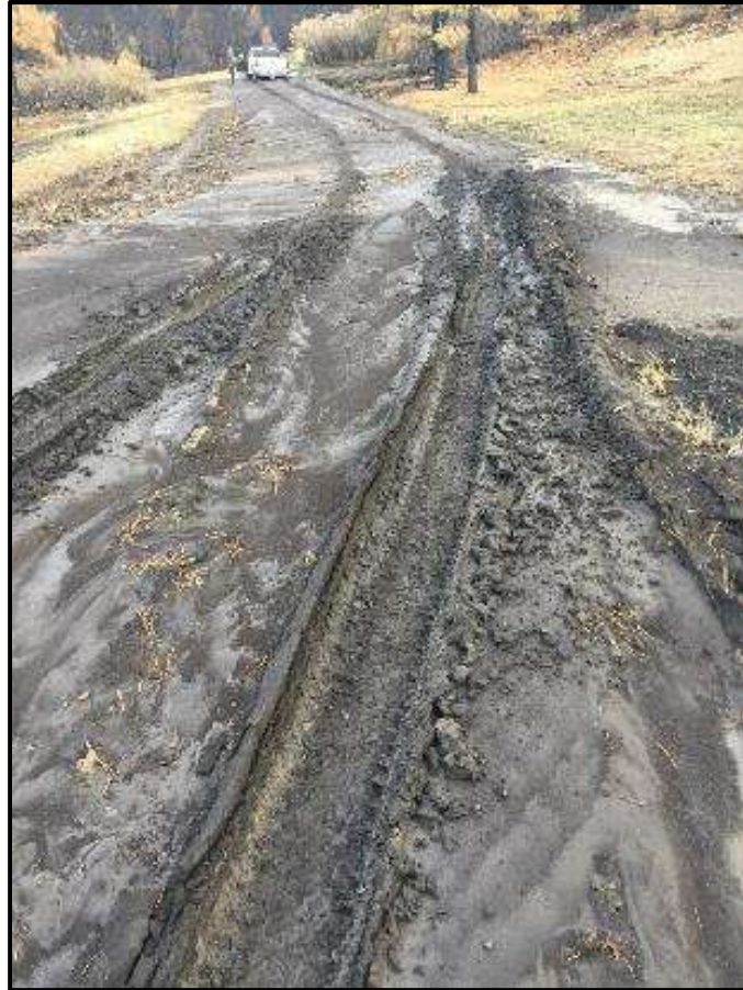
Figure 3.65. Post-fire flooding and sediment flow impacts to road surface in Philmont Scout Ranch.
