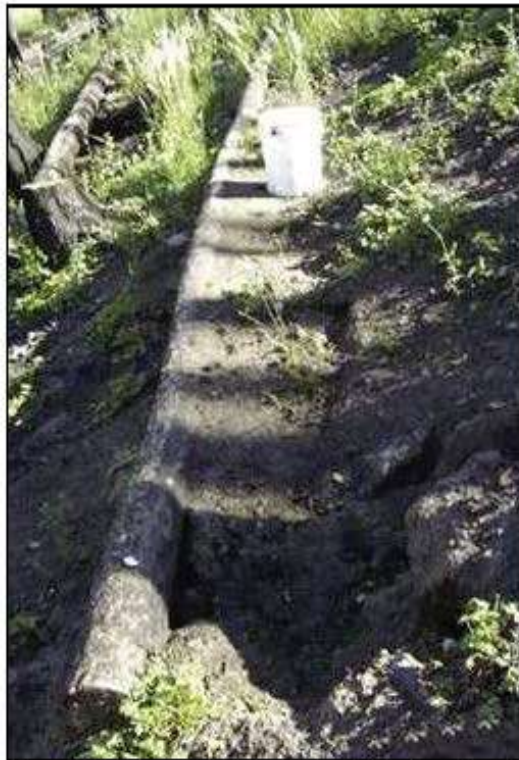
Figure 20—Contour-felled LEB which has filled with sediment and then failed. Sediment trapping ability of LEBs on steep slopes is limited.
