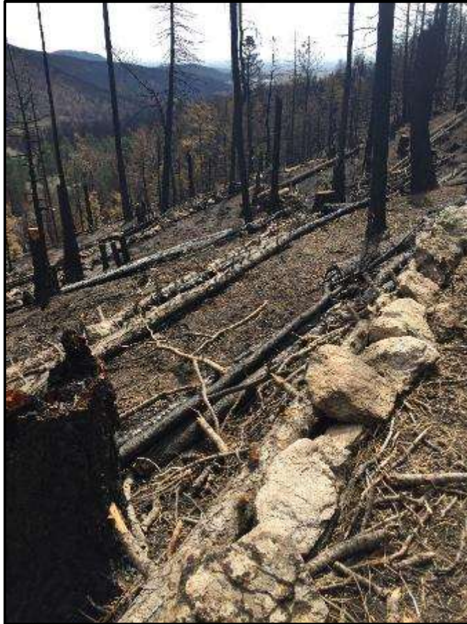
Figure 3.43. Log erosion barriers installed above Cimarroncito intake structure on Philmont Scout Ranch.
