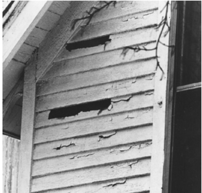
Figure 15–15. Paint can peel from wood when excessive moisture moves through house wall. Some cross-grain cracking is also evident on this older home.
