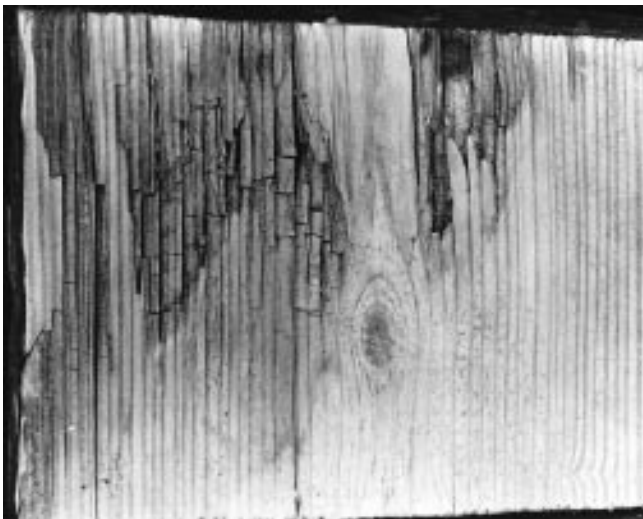
Figure 13-5. Brown rot in Southern Pine railroad tie. Note the darker color and the cubical checking in the wood.
