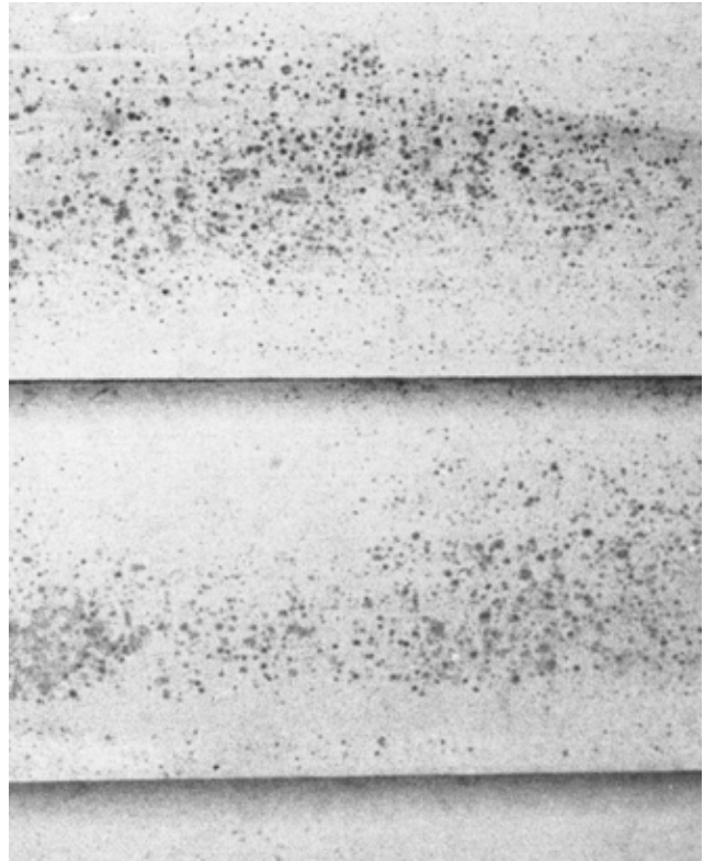
Figure 15-18. Mildew is most common in shaded, moist, or protected areas.
