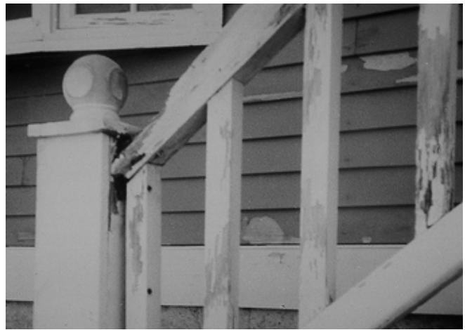
Figure 15-10. Decay in wood railing fully exposed to weather.
