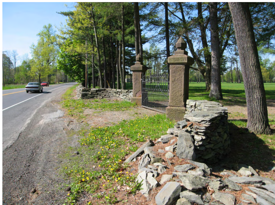
Figure 12: Recent view of the Home Road entrance looking south along the Post Road showing deteriorated condition of road shoulder, earthen roadbed, and stone wall. (SUNY ESF, 2007.)
