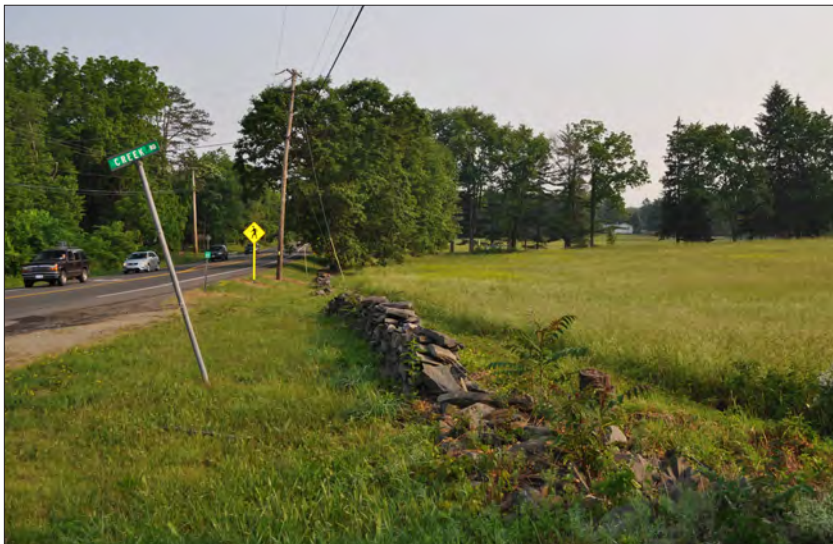
Figure 3.8. Collapsed and buried sections of stone wall at the front of Val-Kill, looking north along Violet Avenue, 2011. (Olmsted Center for Landscape Preservation)
