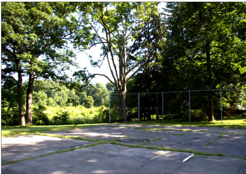
Figure 2.1: Looking northeast at the tennis court, 2010. This shows the poor condition and missing components (net) that contrast with the historically well-maintained and lively character of the landscape. (Olmsted Center for Landscape Preservation)
