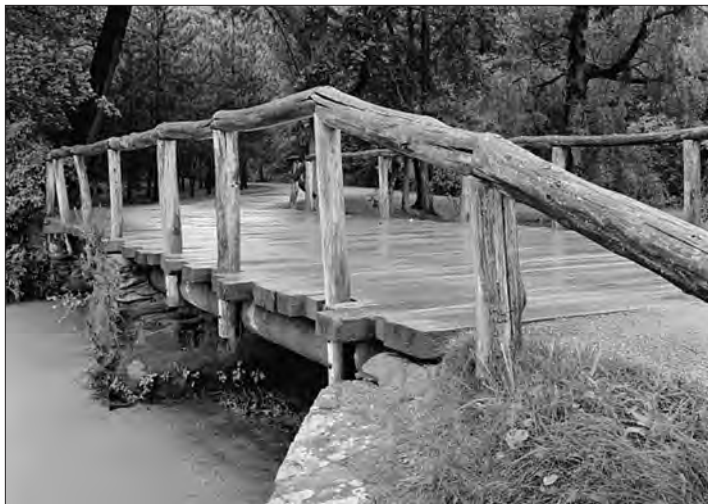
Figure 3.34. Rustic railings on the Fall Kill bridge that most likely date to the 1950s, photographed 1978. (Historic American Building Survey, NY-5666)
