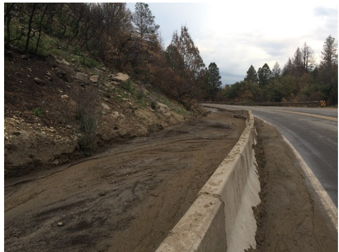
The New Mexico Department of Transportation utilized concrete K-rails to reduce sediment washing off the Ute Park Burn on Highway 64 west of Cimarron, NM. © Mary Stuever/NMFD
