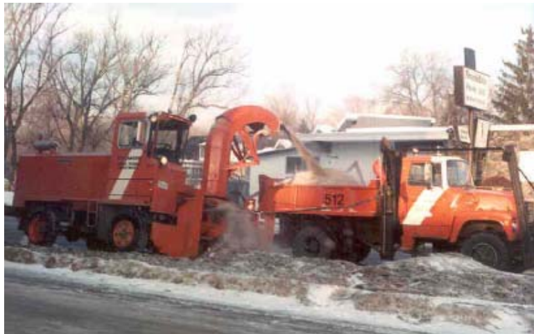
Using a snow blower to load trucks of hauling contaminated snow banks ( http://www.ogra.org/lib/db2file.asp?fileid=9198 )
