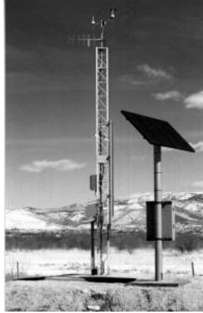
Remote Weather Station (Federal Highway Administration 2004)
