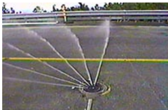
Example of in roadway sprinkler head (Ministry of Transportation 2001)
