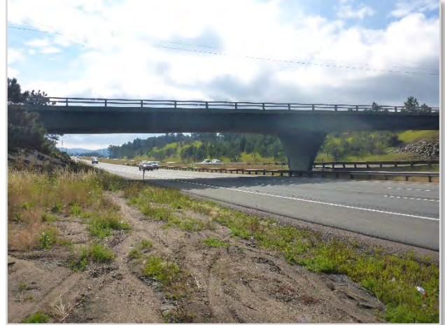
Photo 6. Looking west from the east side of the Beaver Brook/Floyd Hill interchange bridge over I-70 during the Summer of 2017.
