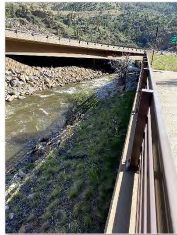
Photo 24. Picture looking east along East Idaho Springs Road west of the Hidden Valley/Central City interchange near MP 242.7 in May of 2020. Shows the narrow riparian corridor and the steep riprapped banks.
