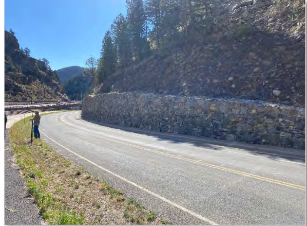
Photo 22. Looking east from East Idaho Springs Road/I-70 Frontage Road at the forested southern slopes with retaining walls. Very little vegetation present in a grassy area between the road and the Clear Creek Greenway. Near MP 242.5 in May 2020.
