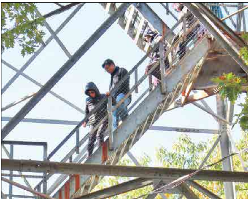
Algonquin Highlands council is committed to finding more than $1.3 million if the township is successful in getting a $3 million grant for the Dorset Tower under the Investing in Canada Infrastructure Program. File.
