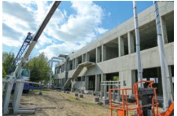
Construction of the office building took 4 years – the picture presents assembly of the terrace steel structure. 2014
