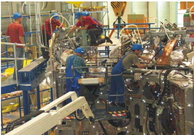
Figure 19: Trial assembly of bus-bars in the first module
