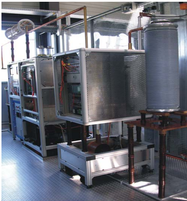
Figure 31: Modulator/heater/crowbar unit installed in the gyrotron hall in Greifswald. The modular structure of the HV-modulator (background), the thyatron crowbar unit with the cathode heater cabinet (centre), and ignition coil for the thyatron (foreground) are shown.
