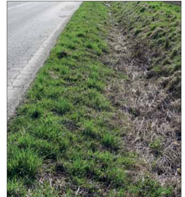
Figure 7.1.11.1 Road side swales. Photo: I. Tichá
