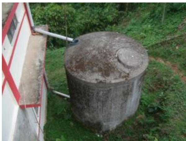
Rain water harvesting tank collecting water from roof top in Bethany Society training center, West Garo Hills District
