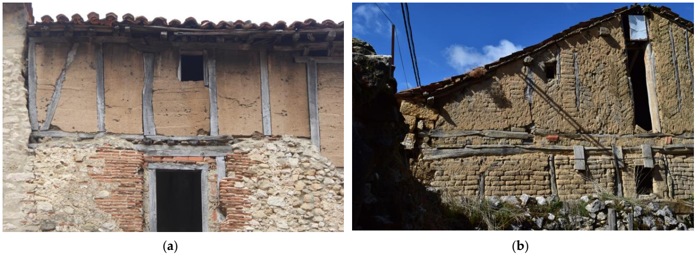
Figure 1. Examples of half-timber walls with heavy infills: (a) monolithic infill of gypsum concrete in Pancorbo (Burgos); (b) masonry infill of adobe infill in Moral de Hornuez (Segovia).
