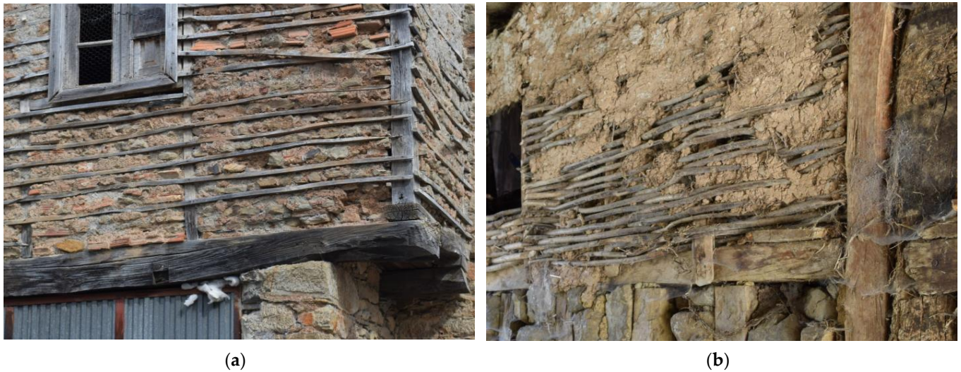
Figure 26. Half-timber walls with lightweight enclosures executed using wooden elements: (a) lath-and-daub enclosure with laths identified as Alnus glutinosa L. in Almagarinos (León); (b) Wattle-and-daub enclosure with flexible rods identified as Corylus avellana L. in Caloca (Cantabria).
