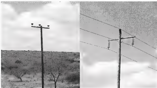
Figure 1a & b. 1a (on the left) shows the typical “T-structure” which poses an electrocution risk to birds perching on the cross arm. 1b shows the “inverted T” pole structure which is safer for perching birds since the outer conductors are suspended below the cross arm out of reach of birds.
