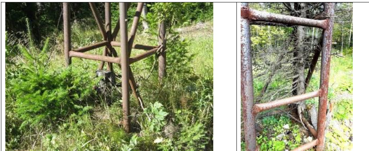
Fig. 77. Cut spruces that settled down among the towers and endangering the high tension lines. They gave place to young optimists. Photo by V. Usoltsev.
