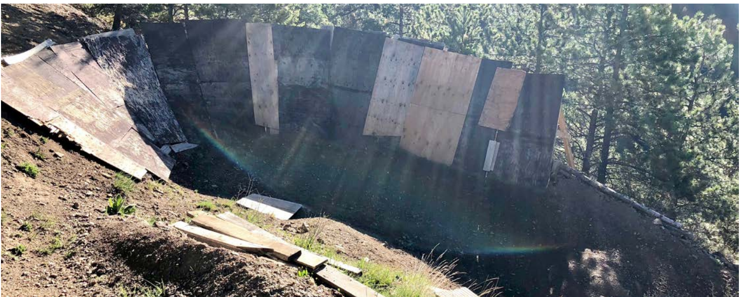
Existing Dilapidated Rogue Trail Features
