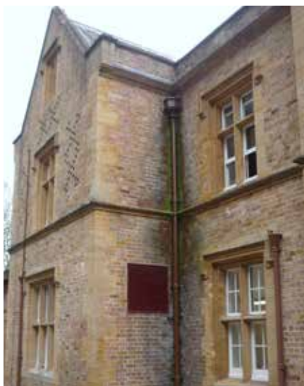
Insufficient guttering on Norton Manor, a Grade II listed building © Crown
