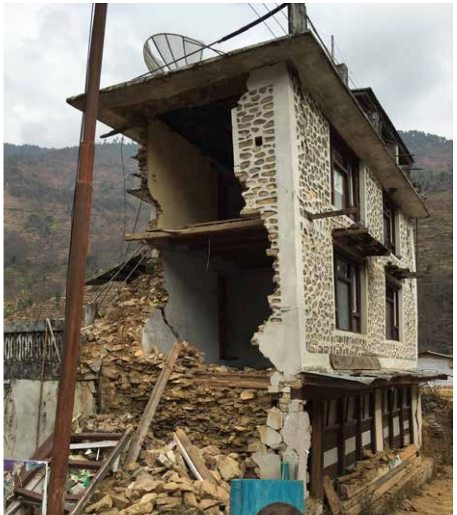
Earthquake damage © Crown
