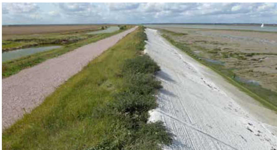
Example section of priority sea defence repairs and improvements, showing the enhanced access track, retained vegetation where possible and new concrete revetments. New rock toe-protection, and raised sea defences have been installed where necessary to defend against predicted flood risk scenarios © QinetiQ
