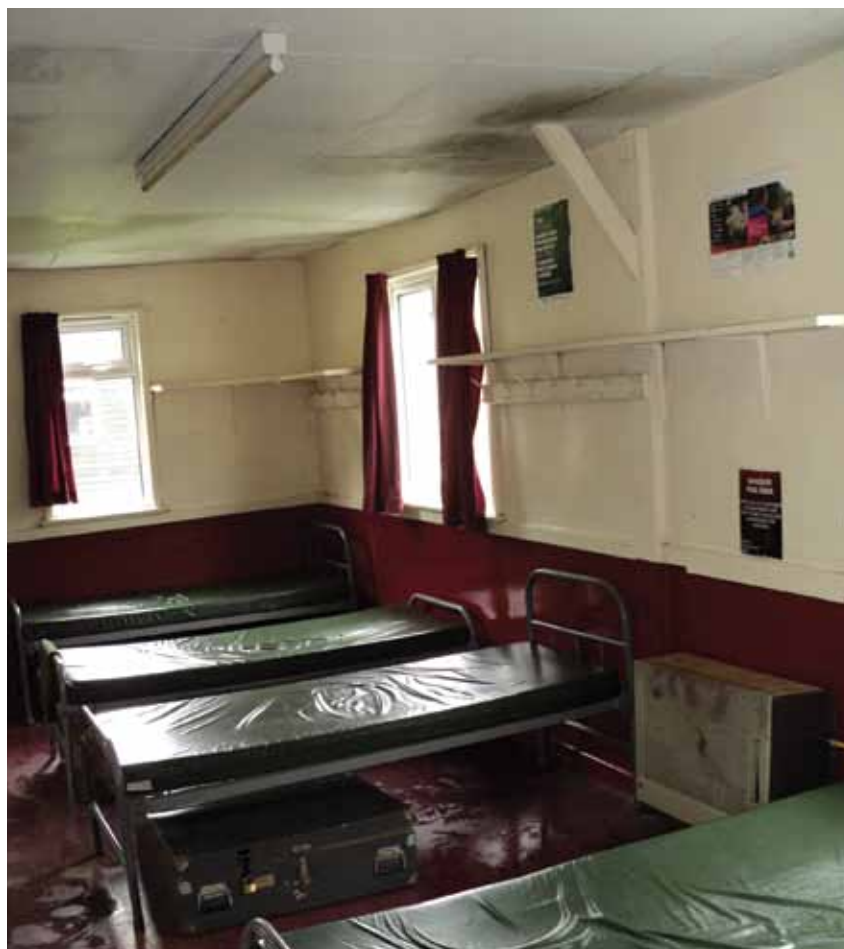
Original timber accommodation hut showing Drugasar heaters, poorly insulated suspended ceiling and un-insulated walls © Landmarc
