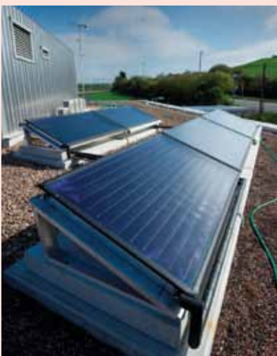
Solar panels one of the projects many energy saving measures © Debut
