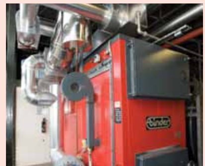
Biomass boiler on a military establishment © Debut
