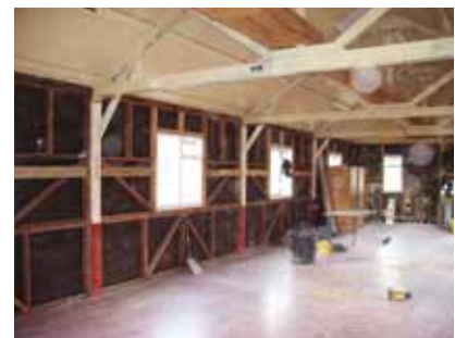
Stripped out timber hut showing timber frame and roof structure above suspended ceilings © Landmarc
