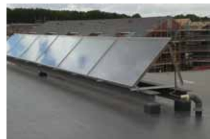
Solar thermal heating solutions at Assaye Barracks, Tidworth © Project Allenby/Connaught
