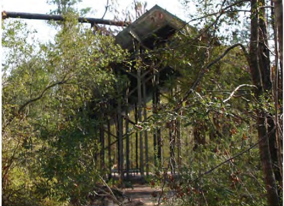
The Pinecote Pavilion at the Crosby Arboretum suffered significant damage caused by Hurricane Katrina's high winds and the falling of nearby trees.
