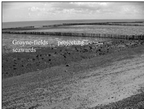
Fig. 5. Groynes built to form polder-like structures on the foreshore as part of an attempt to 'hold the line', Cudmore Grove, Mersea Island, Essex (at the time the picture was taken in 2003, some 10 years after construction, there were no obvious signs of mudflat accretion or saltmarsh development).
