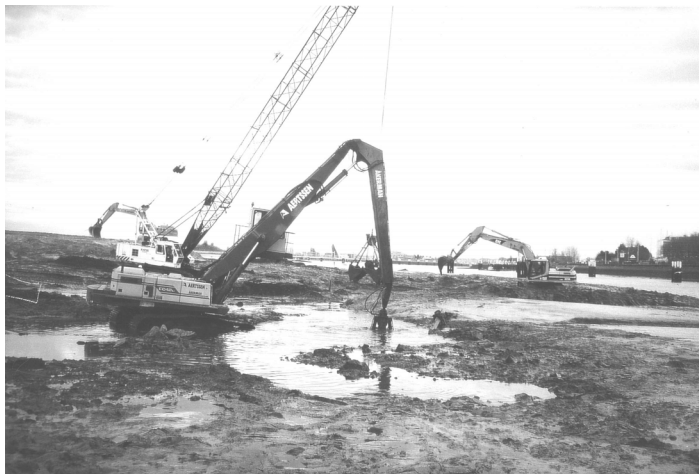
Fig. 5. Phase 2: the 'wet works' or the removal of the jetties and quays of the former Military harbour.
