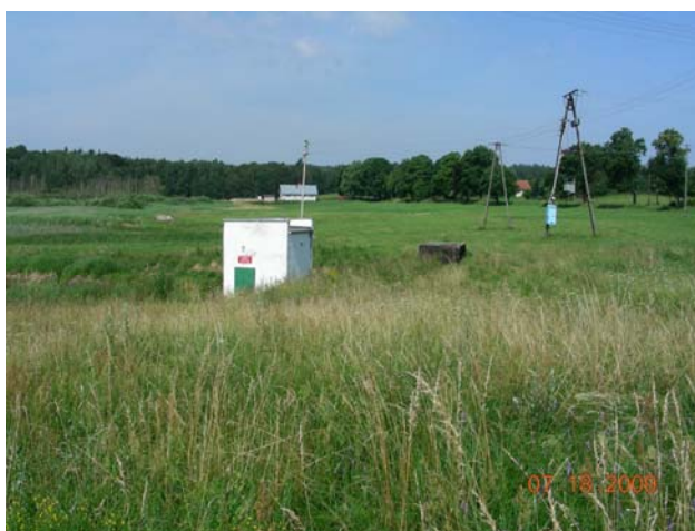
Fig. 7. Pumping station on Gązwa gytja land
