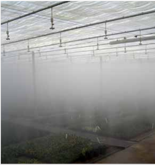
Fog/misting system in the propagation unit
