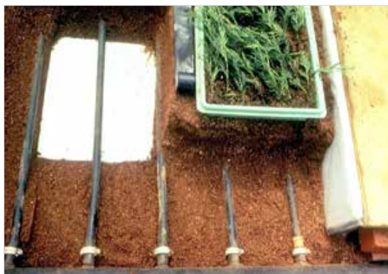
Basal heat provided by piped hot water
