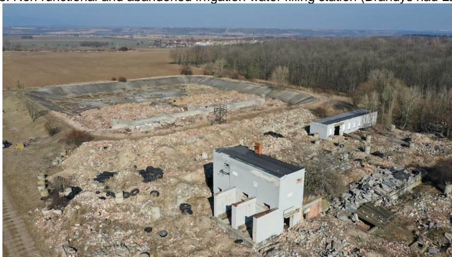
Fig. 9: Non-functional and destroyed irrigation water reservoir and water filling station (Rakovník)
