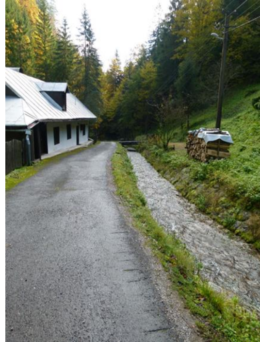
Fig. 3: Reinforced bed of Jelenec torrent in the immediate vicinity of recreational path
