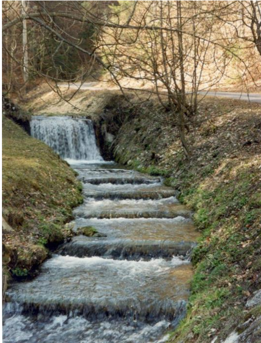
Fig. 2: Weir and sills in Jelenec torrent in the immediate vicinity of the hiking trail
