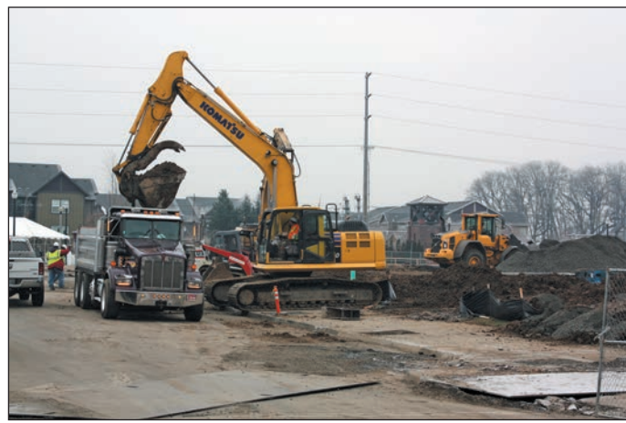
HILLSBORO TRIBUNE PHOTO: DOUG BURKHARDT On Dec. 12, the Holland Partner Group launched its latest Platform District project at Orenco Station. A morning groundbreaking ceremony formally kicked off construction of the Central Podium and East Podium, which will encompass 379 apartments and 20,000 square feet of retail space. Heavy earth-moving equipment is now at work at the site, which is at the corner of Northeast Orenco Station Parkway and Northeast Cherry Drive, adjacent to the MAX line's station at Orenco. A total of three six-story buildings are planned for the parcel.
