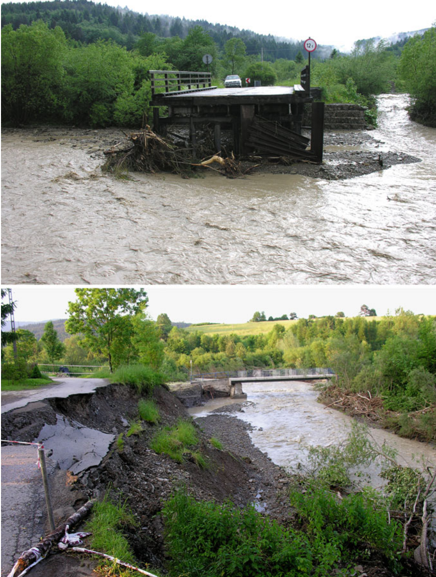
Fig. 2 Damage to infrastructure caused by the 80-year flood of June 2010 on the Biała River. A significant increase in forest cover in the catchment after World War II and widespread in-channel gravel mining conducted in the past decades resulted in sediment starvation of the river and thus the flood action was mainly directed on erosion of the channel boundaries
