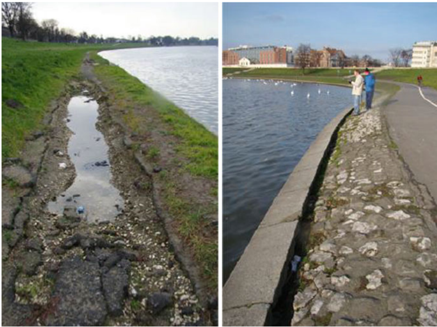
Fig. 6 Destruction of the low boulevard of the River Vistula in the vicinity of the Dębnicki Bridge, in Cracow, resulting of the 2010 flood. Self Source (Politechnika Krakowska)
